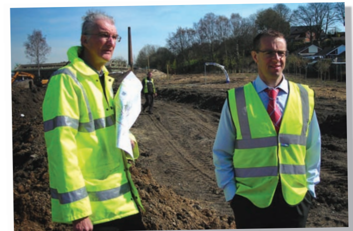
Architect, Tim Nicol of NJL Consultants and Project Manager, Geraint Dodd of P&W Contracting inspect progress
