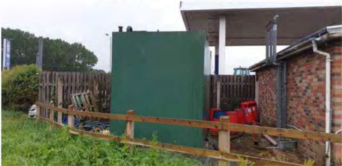
Photo 8: Redundant storage tank on site. No visible signs of spills or leakage identified during the site visit.
