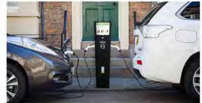
Figure 53; Incorporate Electric Car Charge Points, Image Source: Roltec
