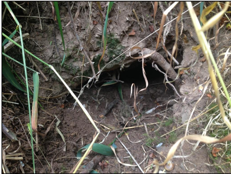
Plate 5. Large hole present at the western end of southern site boundary
