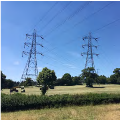
1. FROM B4373 NEAR DUNGEGROVE FARM LOOKING ALONG OVERHEAD LINE TO THE WEST
