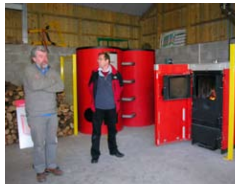
New log boiler, National Trust Cardingmill Valley
