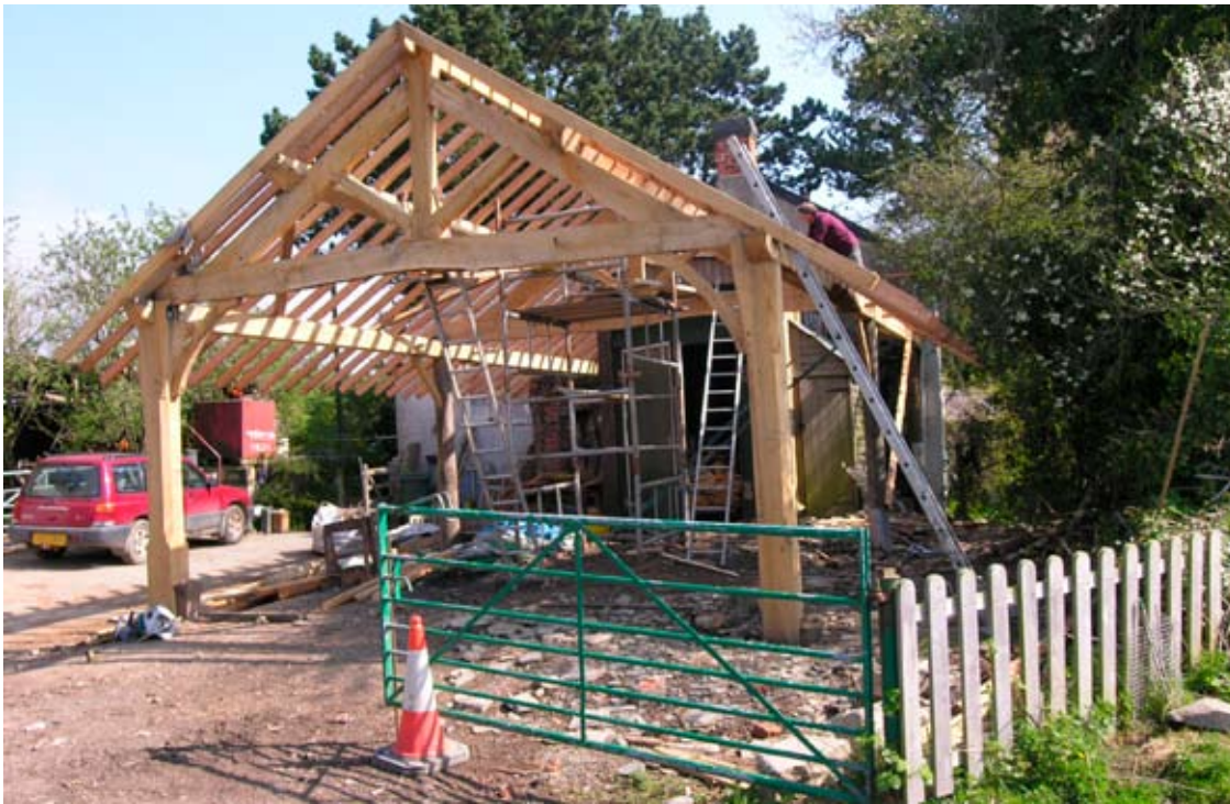
Timber drying shed for Shropshire Hardwoods, an expanding local business, supported by an AONB grant.
